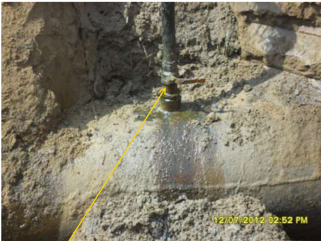
Close up: Illegal fitting on 28" Nkpoku-Bomu pipeline at Gio. Picture was taken during Joint Investigation of 12 th July 2012.
