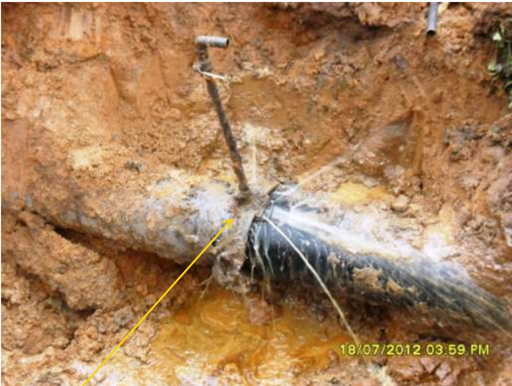
Close up: Illegal fitting on 12" Imo River2 – Ogale pipeline at Owaza. Picture was taken during Joint Investigation of 18 th July 2012.
