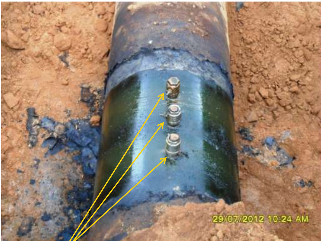
Close up: Illegal fittings on 36" Nkpoku-Bomu pipeline at Atali. Picture was taken during Joint Investigation of 29 th July 2012.
