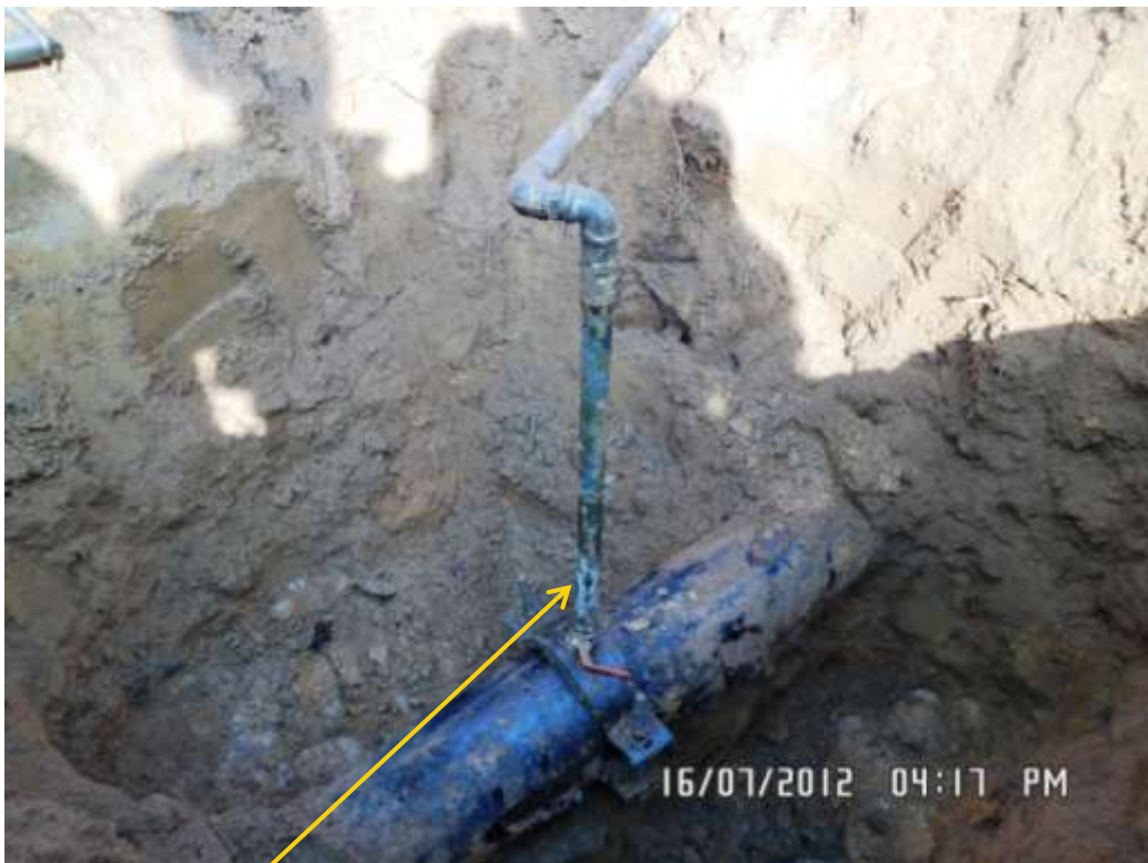
Close up: Illegal fitting on 8" Umuechem-Nkpoku pipeline at Umuwenye- Umuechem. Picture was taken during Joint Investigation of 16 th July 2012.
