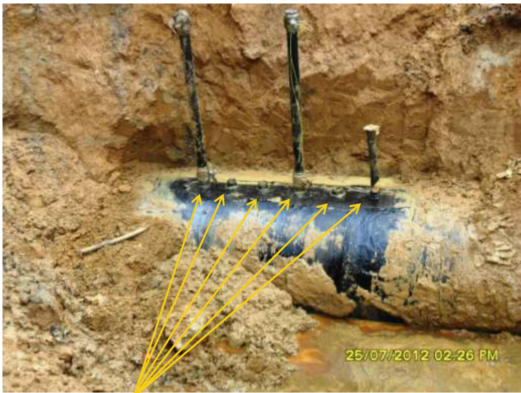
Close up: Multiple illegal fittings on 36" Nkpoku-Bomu pipeline at Eneka. Picture was taken during Joint Investigation of 25 th July 2012.
