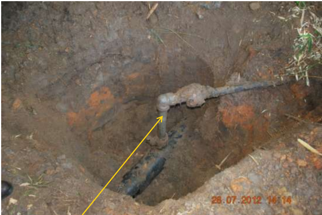
Close up: Illegal fitting on 10" Utorogu-UPS trunkline at Out-Jeremi. Picture was taken during Joint Investigation of 28 th July 2012.
