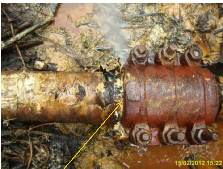
Close-up: Tampered clamp on Well15 flowline at Peremabiri. Picture was taken during Joint Investigation of 15 th February 2012.
