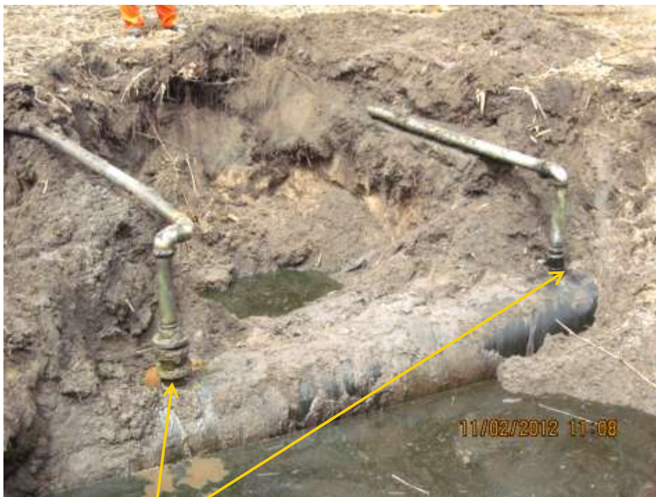
Close-up: Illegal fittings on 28" Npoku-Bomu pipeline at B-Dere. Picture was taken during Joint Investigation of 11 th February 2012.
