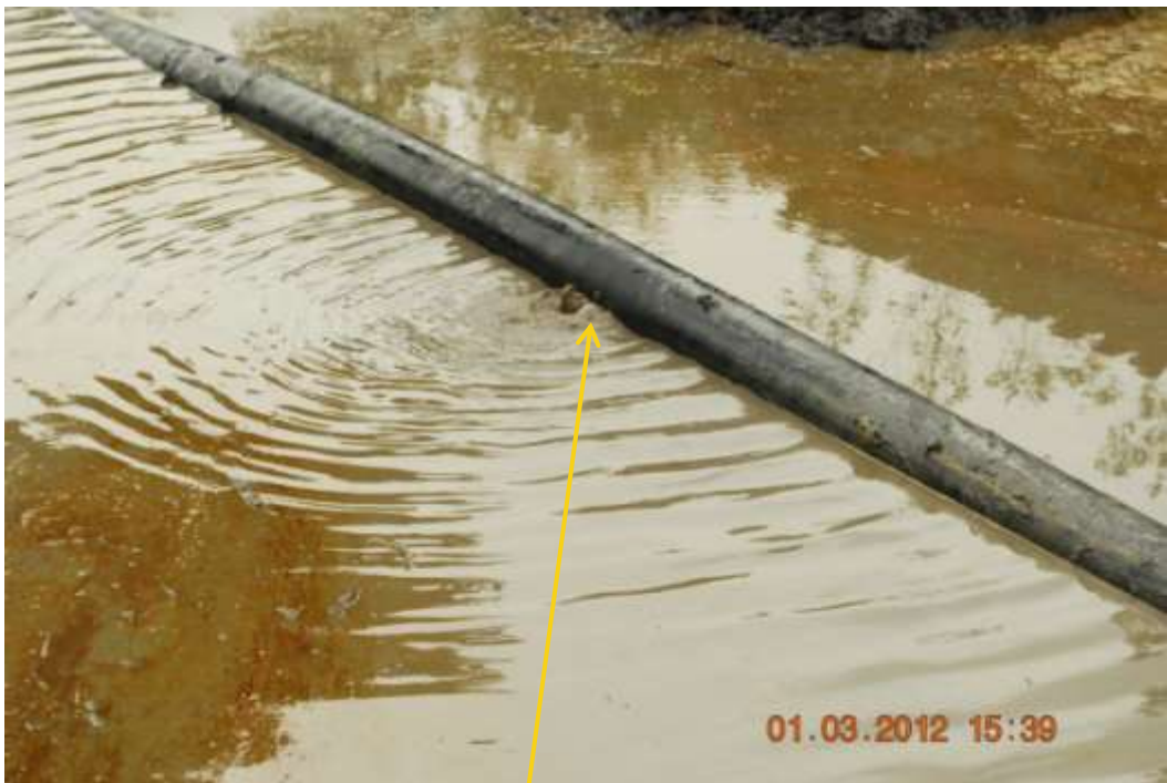
Close up: Spill point on Kanbo Well5 flowline at Egbema-Angalabiri. Picture was taken during Joint Investigation of 1 st March 2012.
