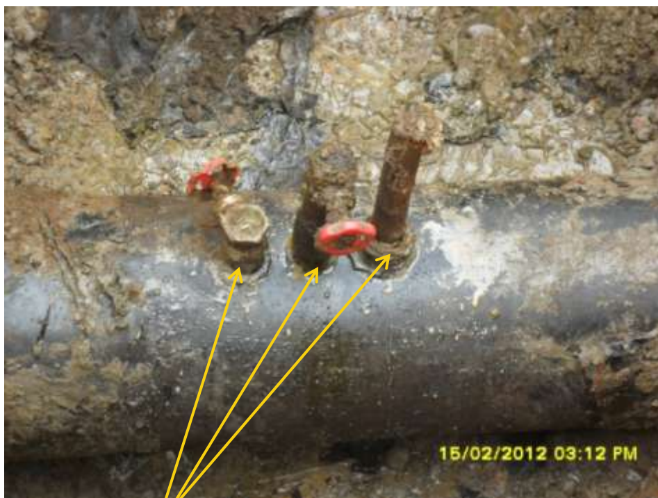
Close-up: Illegal fittings on 12" Imo River2 pipeline at Owaza. Picture was taken during Joint Investigation of 15 th February 2012.
