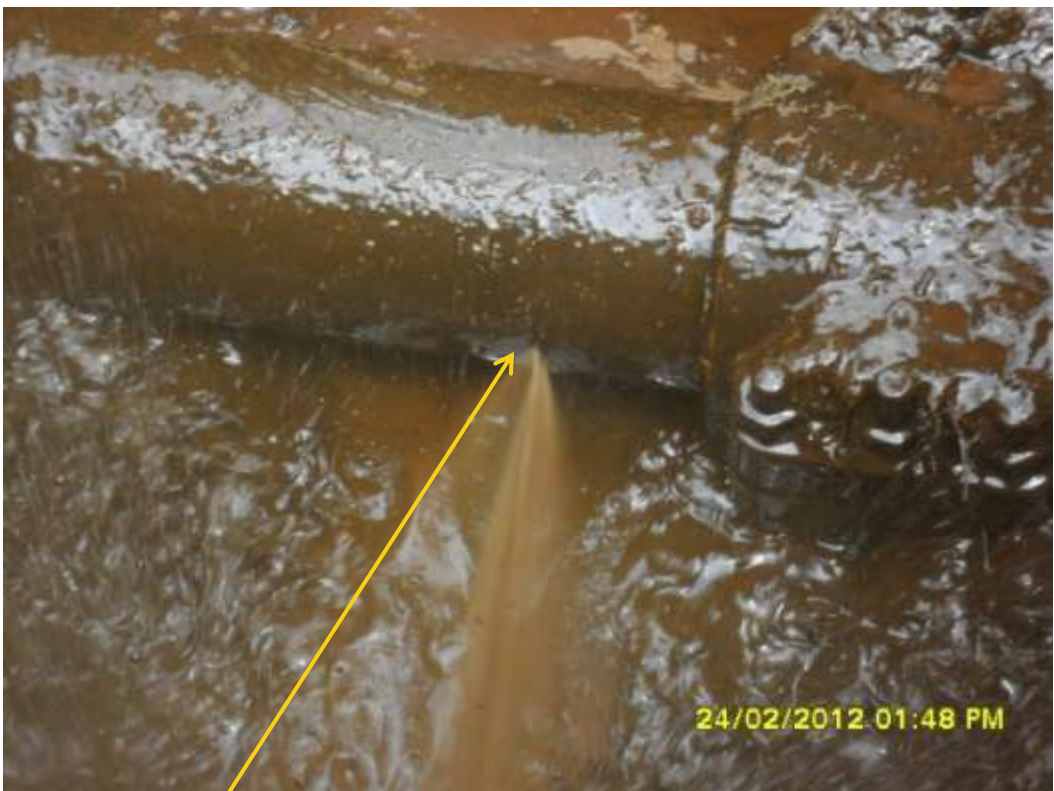
Close up: Spill point on 6" Obigbo north – Ogale pipeline at KomKom. Picture was taken during Joint Investigation of 24 th February 2012.
