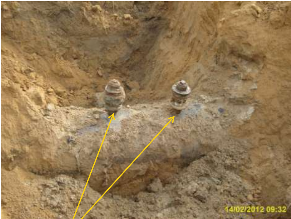
Close-up: Illegal fittings on 28" Npoku-Bomu pipeline at B-Dere. Picture was taken during Joint Investigation of 14 th February 2012.
