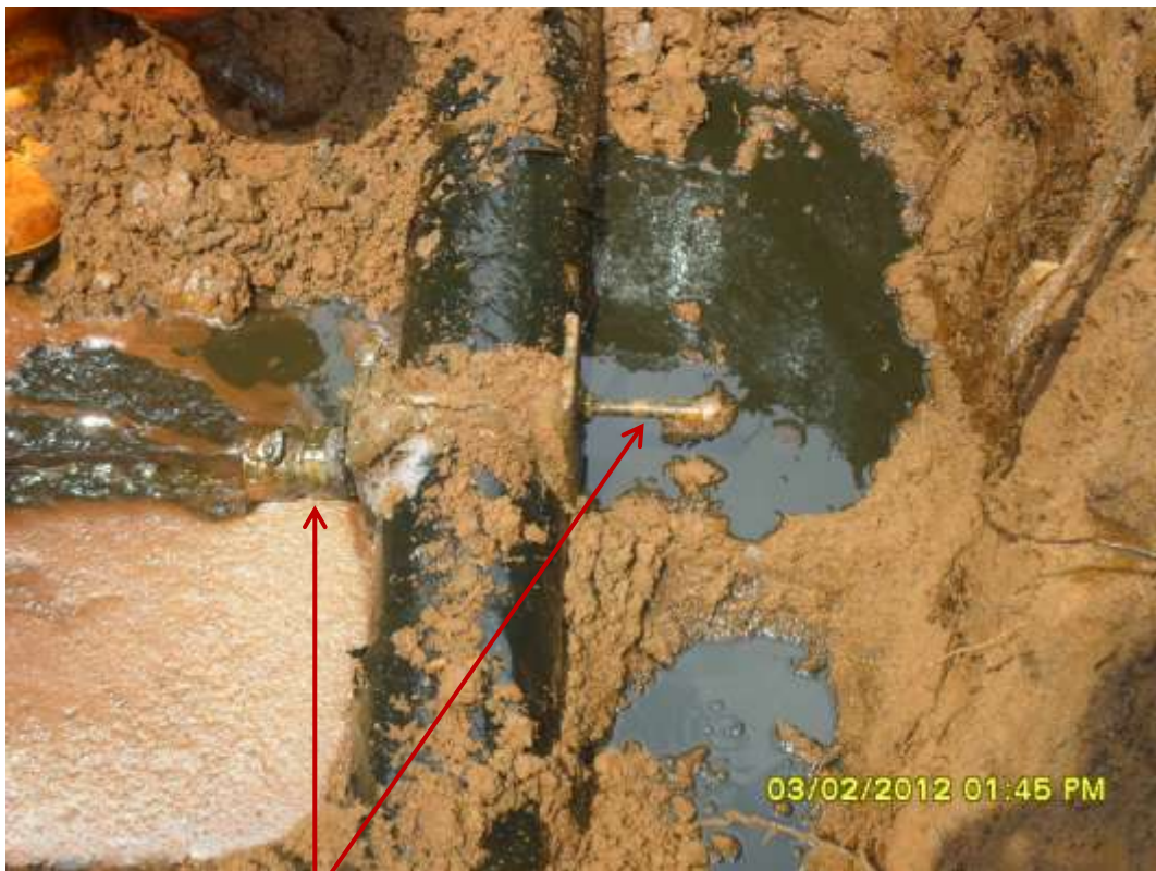
Close-up: Illegal fittings on 6" Obigbo North pipeline at Ogale. Picture was taken during Joint Investigation of 3 rd February 2012.
