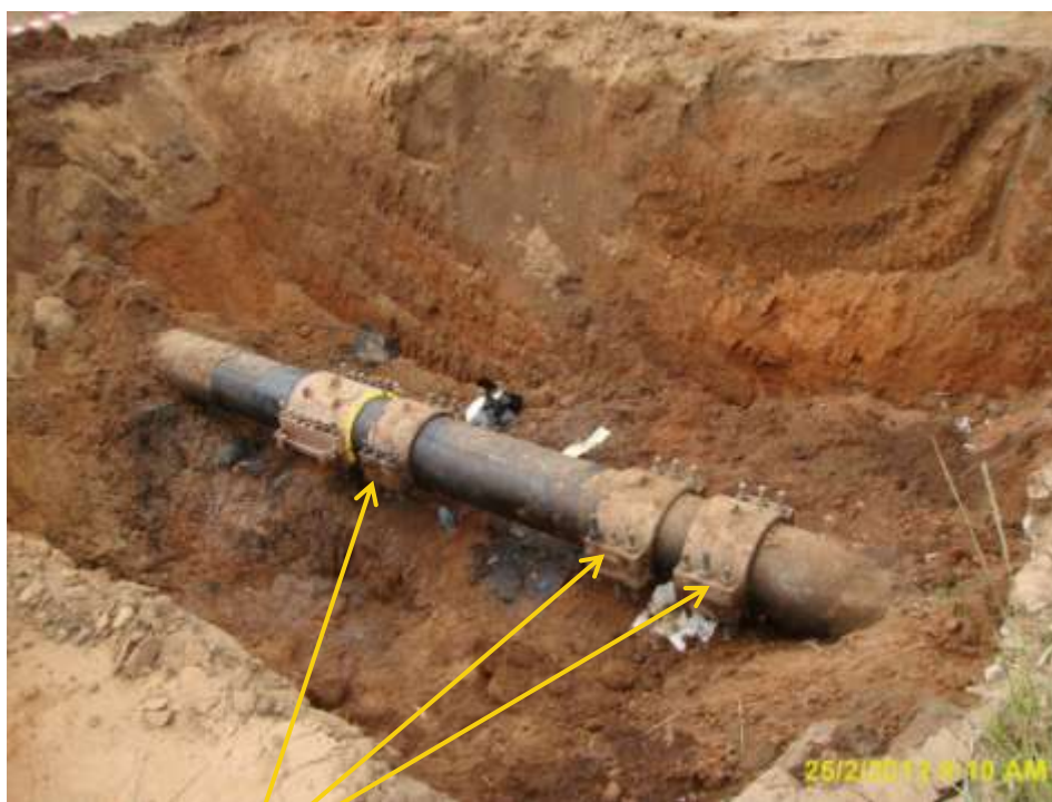
Close-up: Failed clamps on 18" Assa-Rumuekpe pipeline at Awara. Picture was taken during Joint Investigation of 25 th February 2012.
