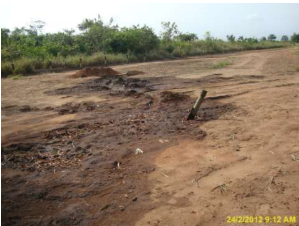
Overview: Part of spill impact on on 18" Assa-Rumuekpe pipeline right of way at Awara. Picture was taken during Joint Investigation of 24 th February 2012.
