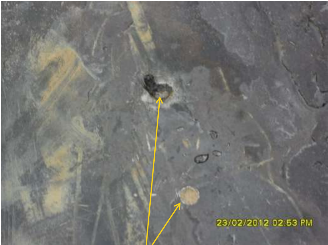
Close up: Drilled holes on 36" Npoku-Bomu trunkline at Agbonchia. Picture was taken during Joint Investigation of 23 rd February 2012.
