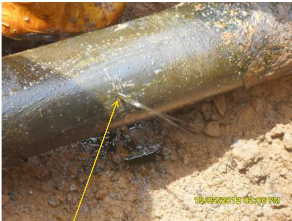
Close-up: Hacksaw cut on 6" Obigbo North – Ogale pipeline at Ogale. Picture was taken during Joint Investigation of 15 th February 2012.
