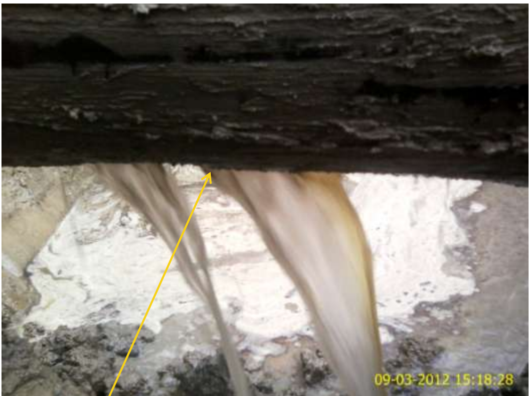
Close up: Tear at 6 o'clock position on 12" Adibawa-Okordia pipeline at Edagberi-Betterland. Picture was taken during Joint Investigation of 9 th March 2012.
