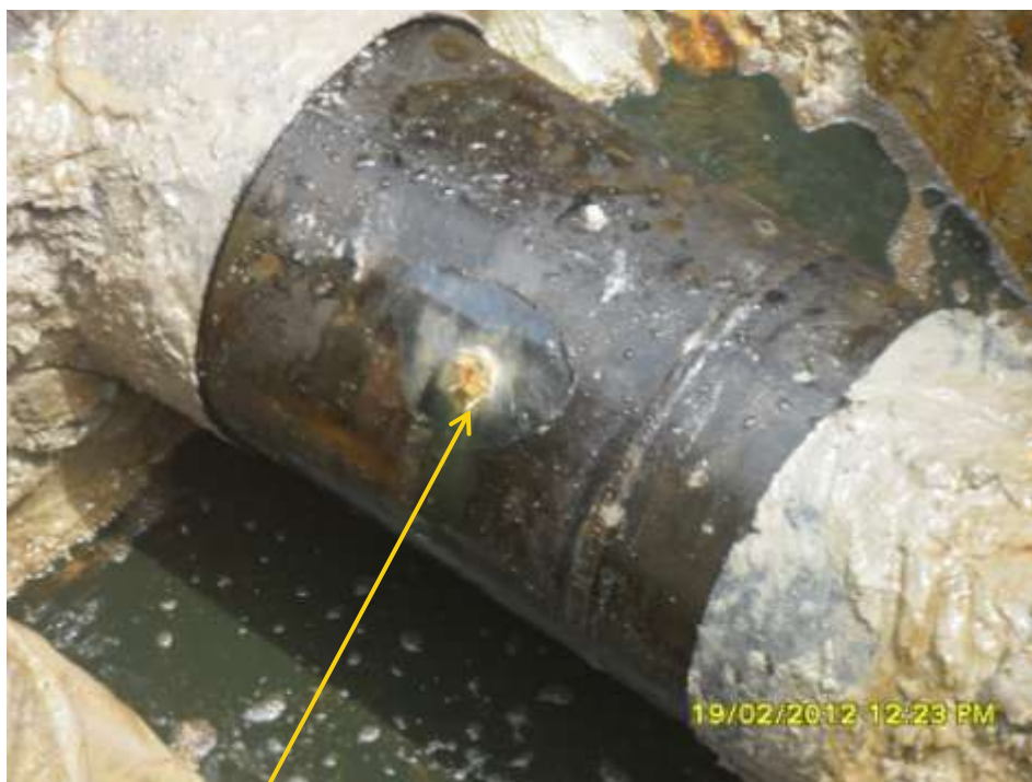
Close-up: Drilled hole on 12" Oguta-Egbema pipeline at Obiakpu. Picture was taken during Joint Investigation of 19 th February 2012.
