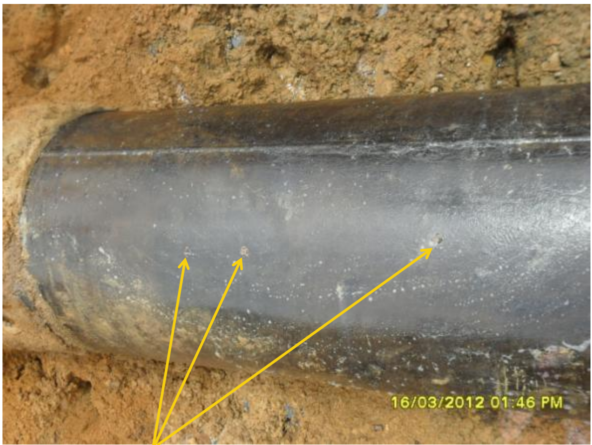
Close-up: Drilled holes on 28" Nkpoku – Bomu Pipeline at Aleto-Nchia-Eleme. Picture was taken during Joint Investigation of 16 March 2012.
