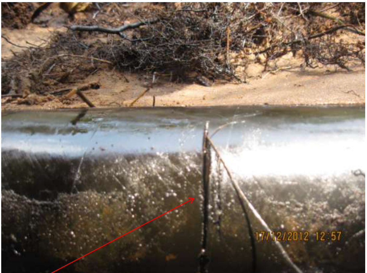
Close-up: Hacksaw cut on 4 inch Otamiri Well 8L Flowline at Umuechem. Picture was taken during Joint Investigation of 17 th Dec. 2012.
