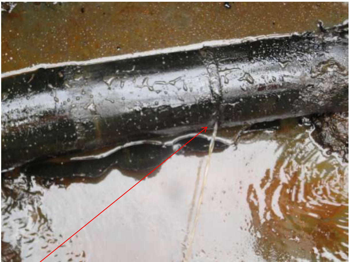
Close-up: Failed weld on Ekulama 2 Well 38L Flowline at Freetown-Kula. Picture was taken during Joint Investigation of 11th Dec. 2012.
