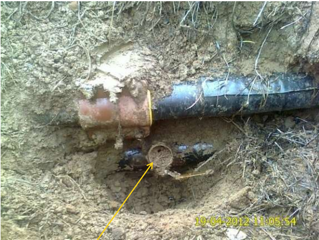
Close up: Illegal fitting on 4" Nkali Well10L flowline at Odagwa2.
