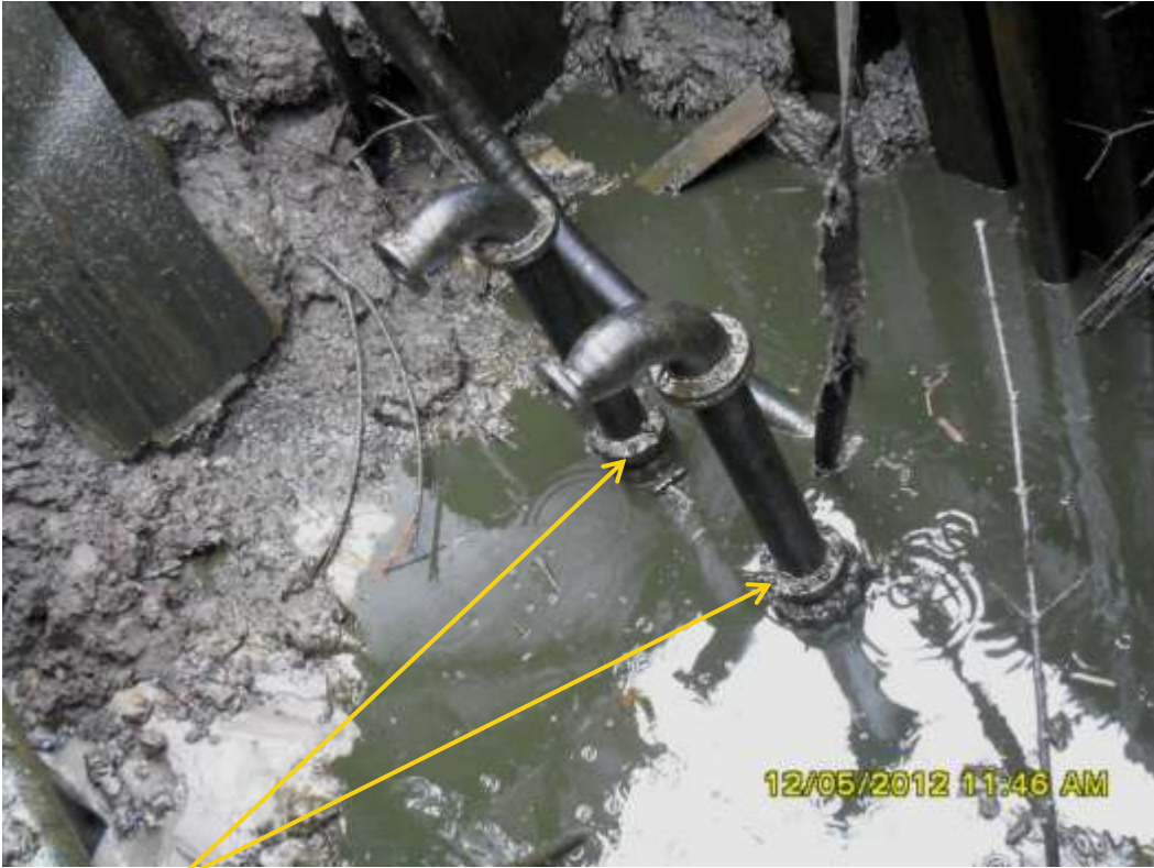
Close up: Illegal fittings on 24" Nembe Creek – Cawthorne Channel trunkline near Tora Manifold at Bassambiri. Picture was taken during Joint Investigation of 12 th May 2012.
