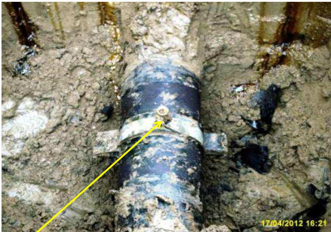
Close up: Illegal fitting on 12" Imo River – Ogale pipeline at Owaza. Picture was taken during Joint Investigation of 17th April 2012.
