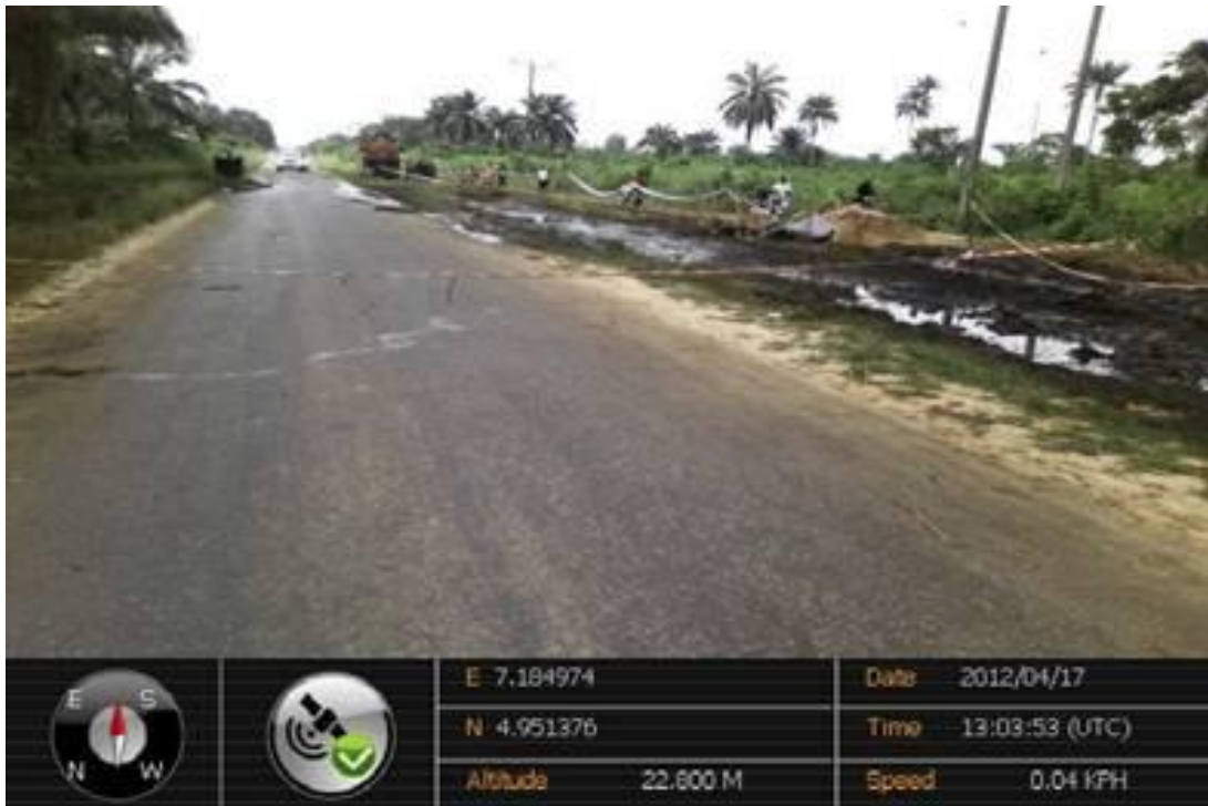
Overview: Part of spill impact on 12" Imo River – Ogale pipeline at Owaza. Picture was taken during Joint Investigation of 17th April 2012.
