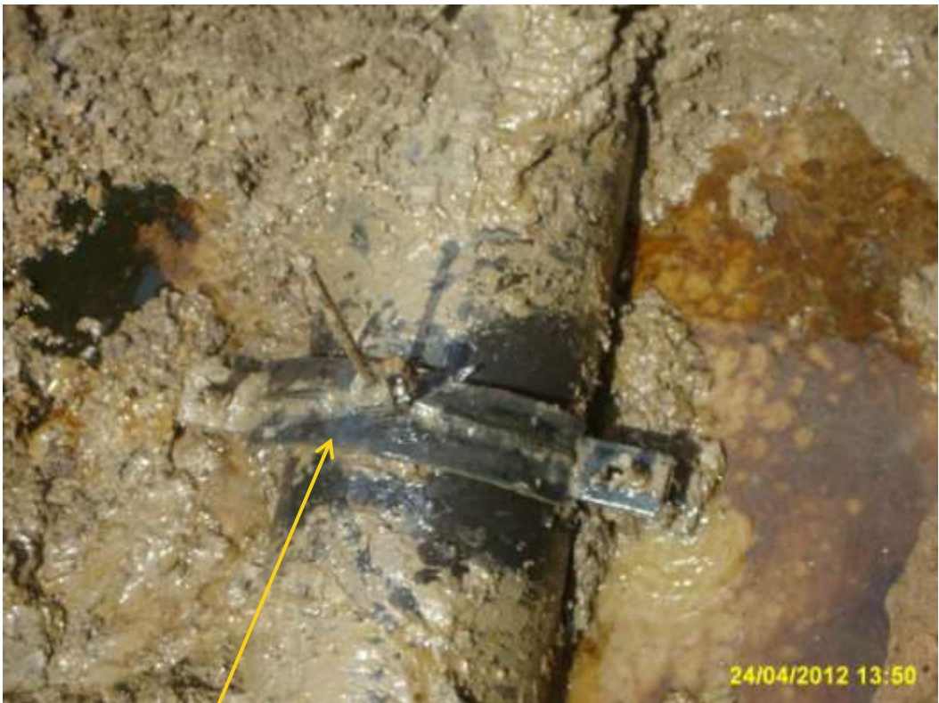
Close up: Illegal fitting on 12" Imo River2 pipeline at Owaza. Picture was taken during Joint Investigation of 24 th April 2012.
