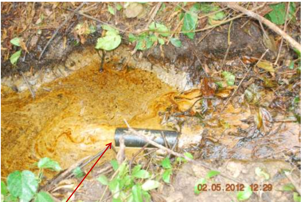
Close up: Cut section on abandoned Oroni Well1 flowline at Enhwe. Picture was taken during Joint Investigation of 2 nd May 2012.
