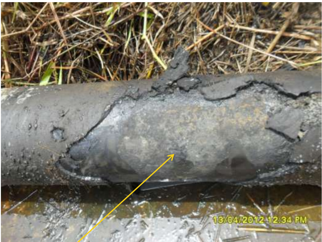
Close up: Evidence of corrosion on 8" Etelebou-Kolocreek pipeline at Biogbolo. Picture was taken during Joint Investigation of 13 th April 2012.
