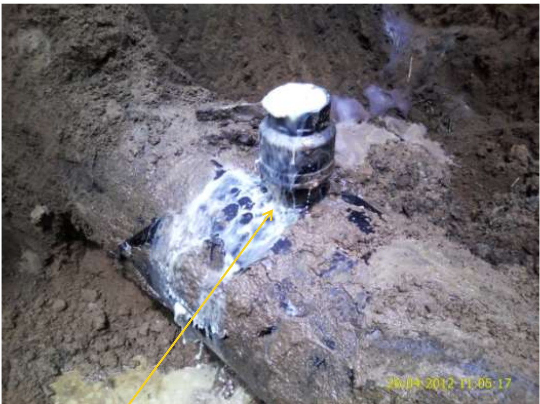
Close up: Illegal fitting on 18" Assa – Rumuekpe pipeline at Awara. Picture was taken during Joint Investigation of 26 th April 2012.
