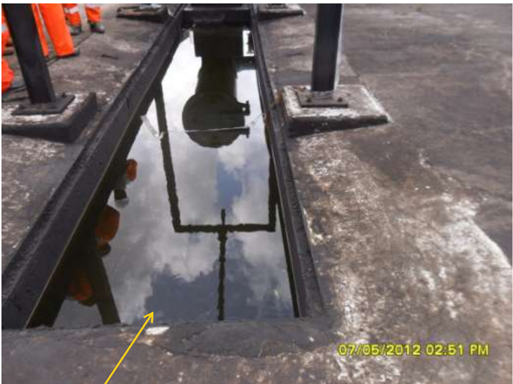
Close up: Saver pit at Bomu Manifold at K-Dere. Picture was taken during Joint Investigation of 7 h May 2012.
