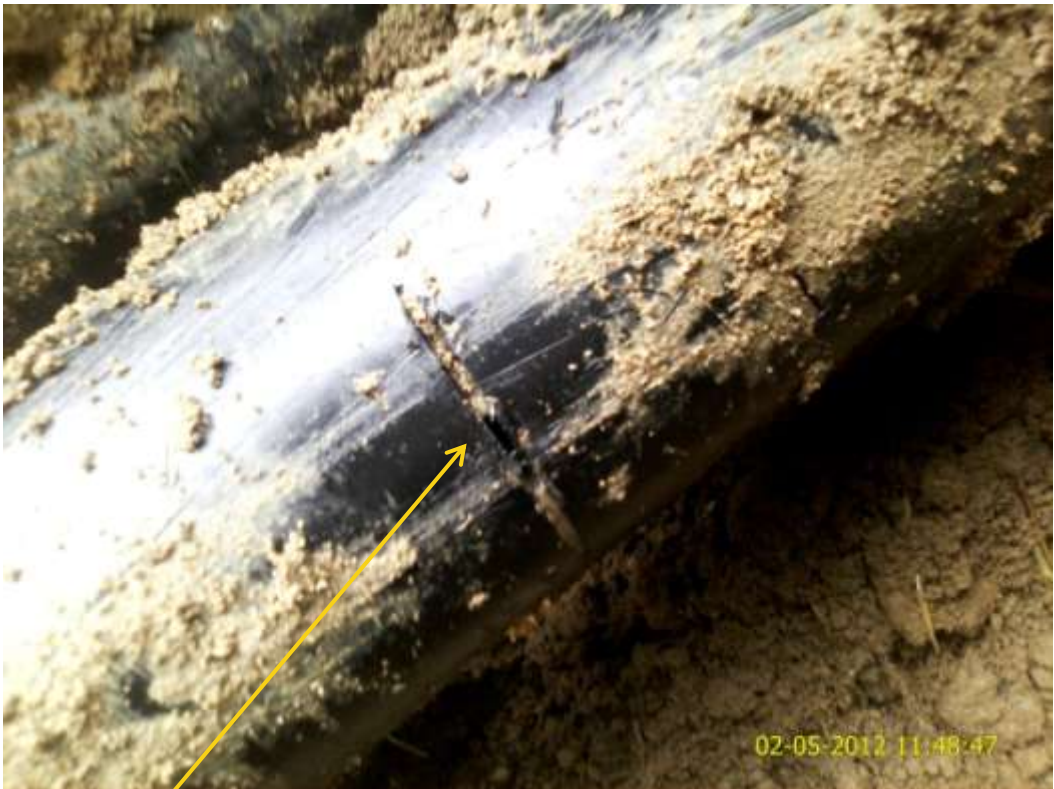
Close up: Hacksaw cut on Ahia Well3S flowline at Omudioga. Picture was taken during Joint Investigation of 2 nd May 2012.
