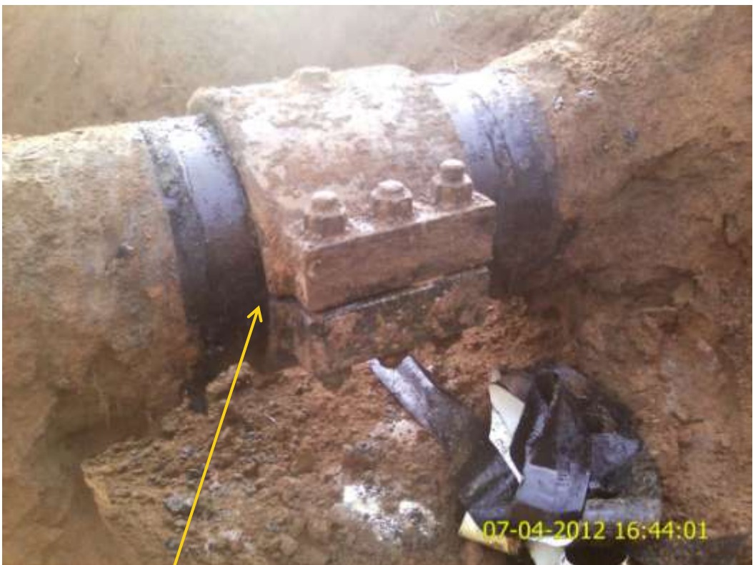
Close up: Failed clamp on 16" Egbema-Assa pipeline at Assa. Picture was taken during Joint Investigation of 7 th April 2012.
