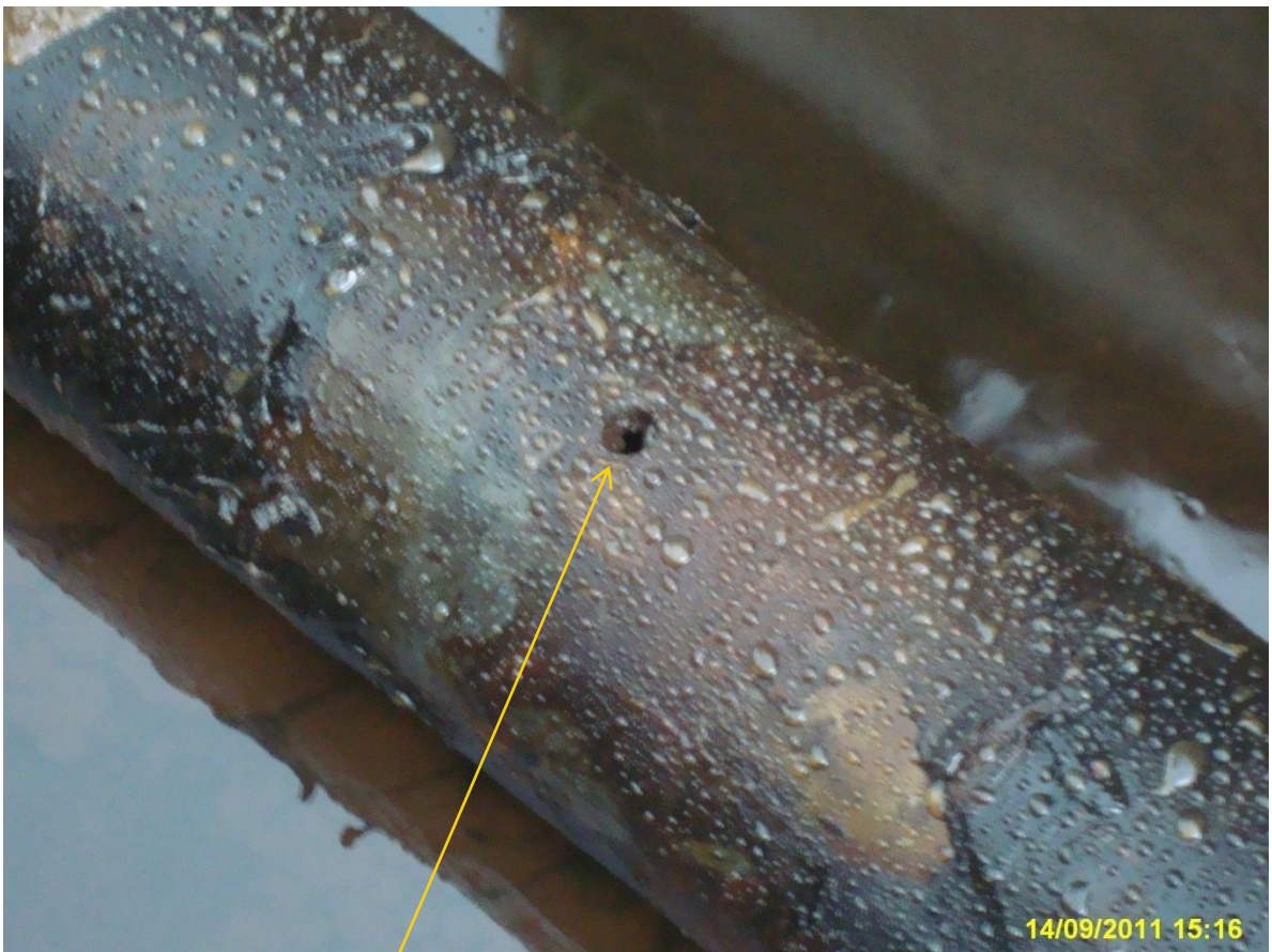
Close-up: Spill due to drilled hole on ImoRiver III Well 1T flowline at Ipu-West. Picture was taken during Joint Investigation of 14th and 15th September, 2011.
