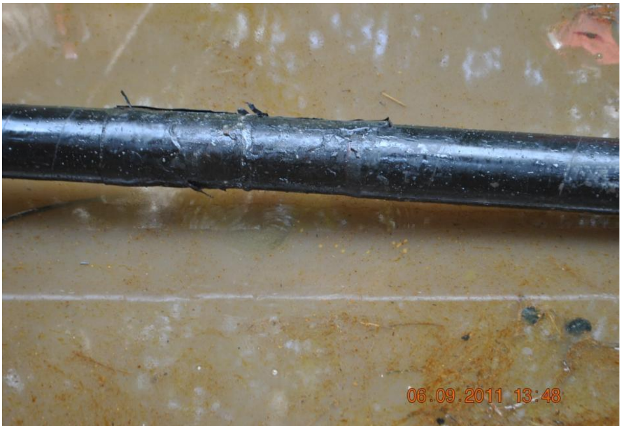
Close-up: Spill due to Internal Corrosion on Opukushi Well 34 Flowline at Agbididama & Egbemo_Angalabiri. Picture taken during Joint Investigation of 6 th September, 2011
