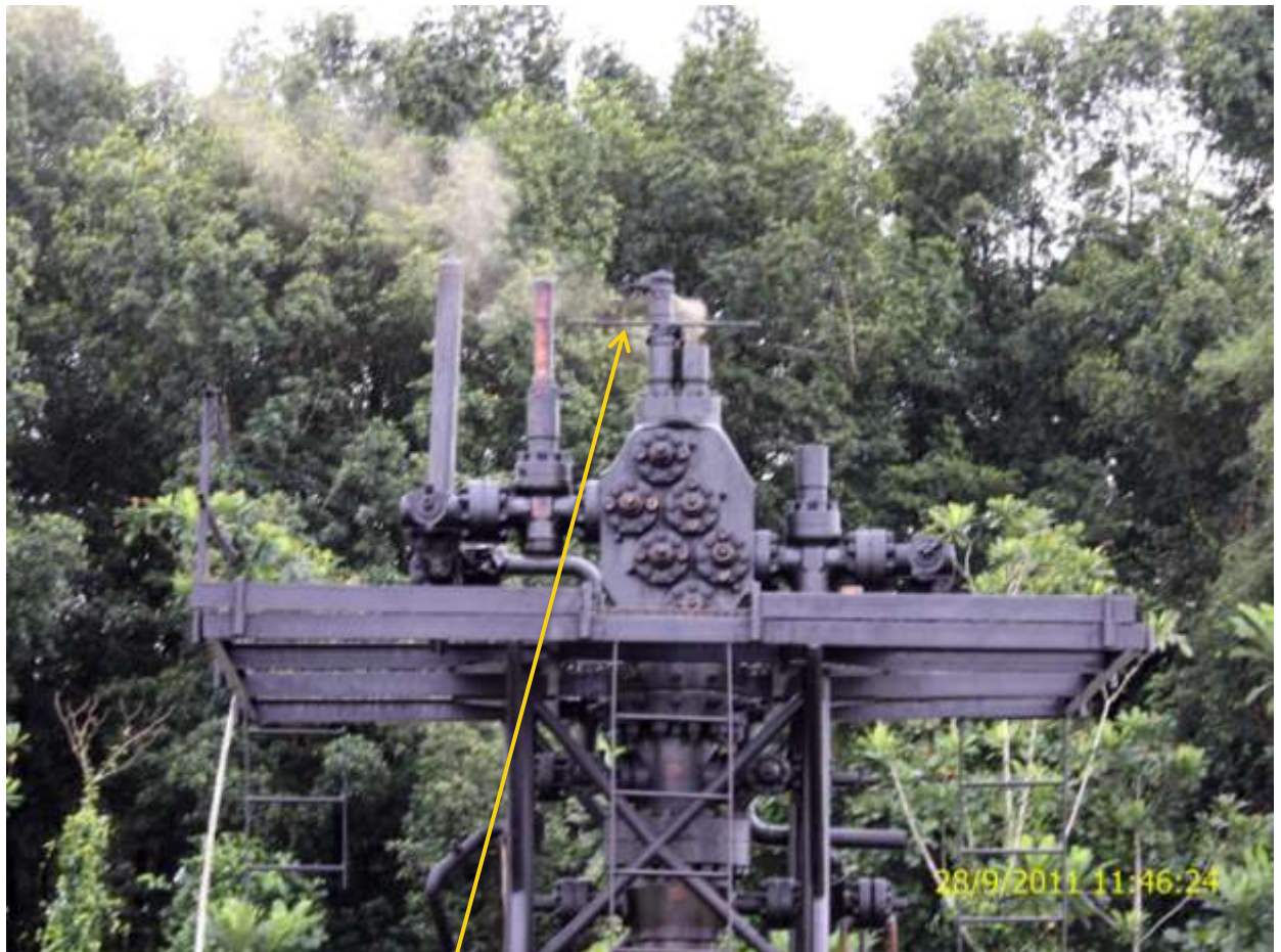
Close-up: Illegal fitting on Jones Creek Wellhead 23SL at Kokodiagbene. Picture taken during Joint Investigation of 20 th September, 2011.
