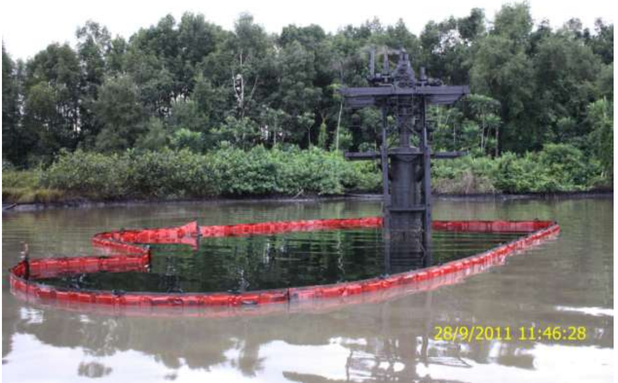
Overview: Part of spill impact on Jones Creek Wellhead 23SL at Kokodiagbene. Picture taken during Joint Investigation of 20 th September, 2011
