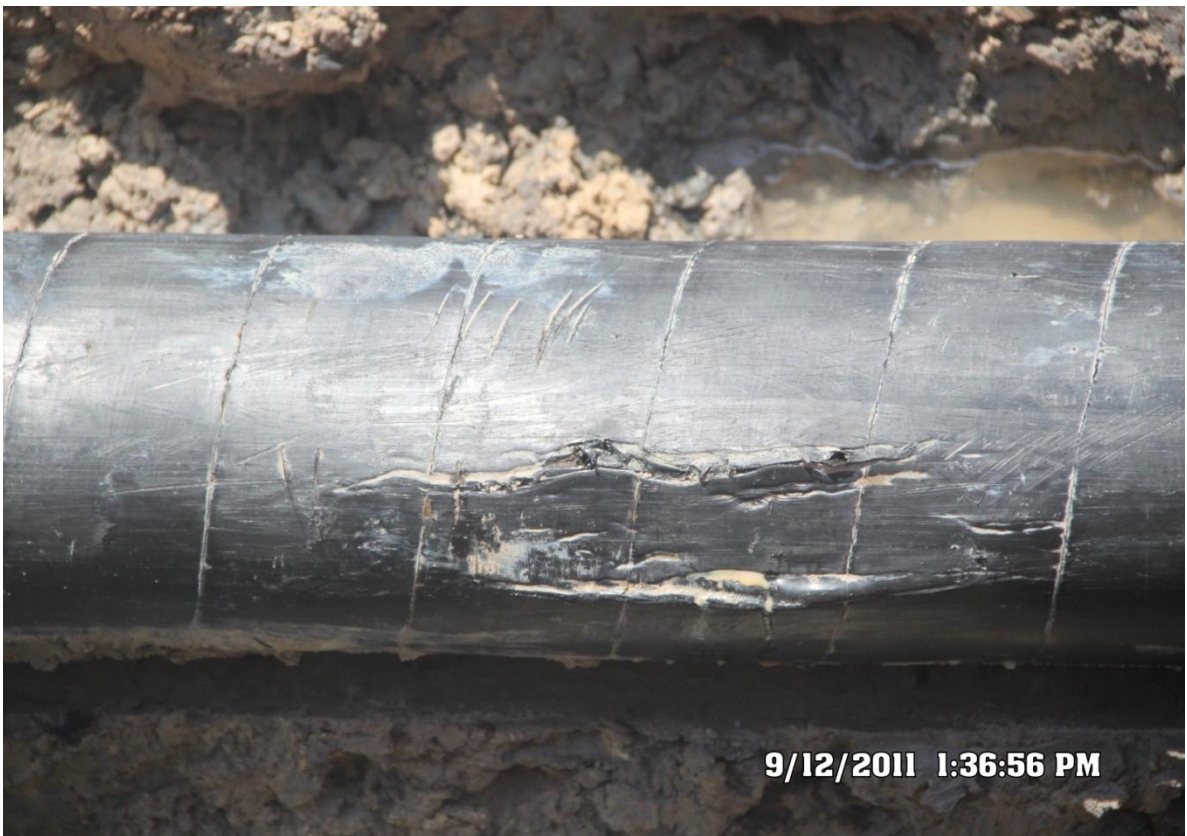
Close-up: Spill due to corrosion on Batan Well 4T 6" Flowline at Batan. Picture was taken during Joint Investigation of 12 th September, 2011
