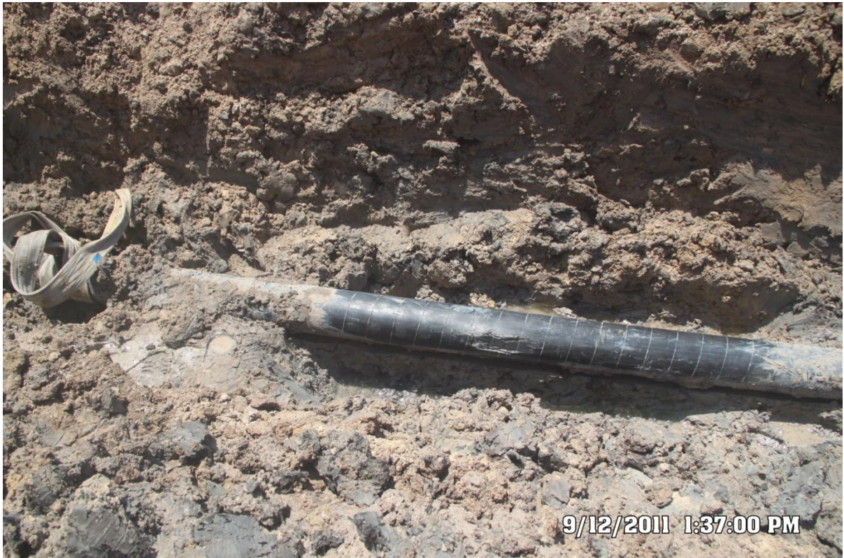
Overview: Part of spill impact on Batan Well 4T 6" Flowline at Batan. Picture taken during Joint Investigation of 12 th September, 2011
