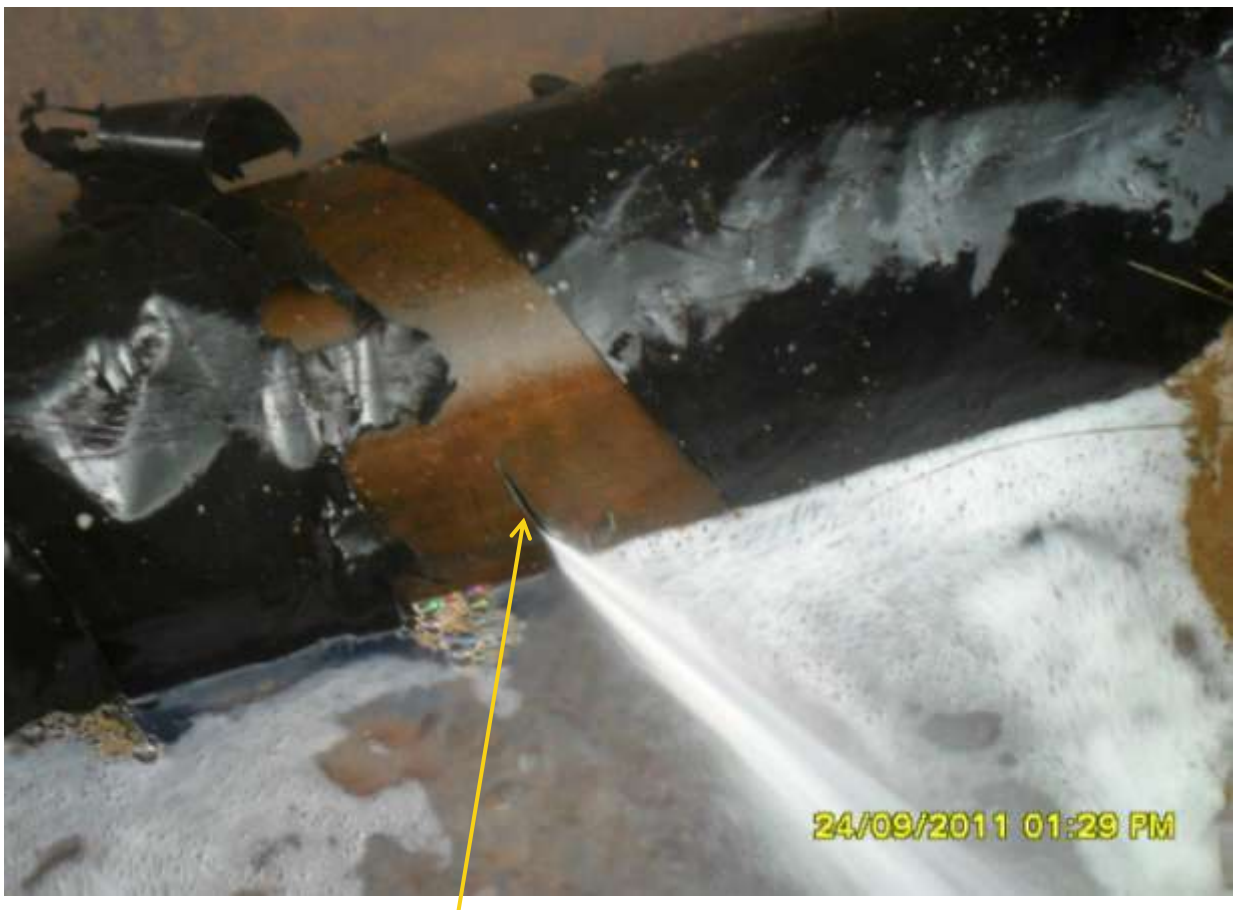
Close-up: Spill point due to hacksaw cut on 6'' Obigbo North-Ogale pipeline at Ogale. Picture taken during Joint Investigation of 24 th September,2011
