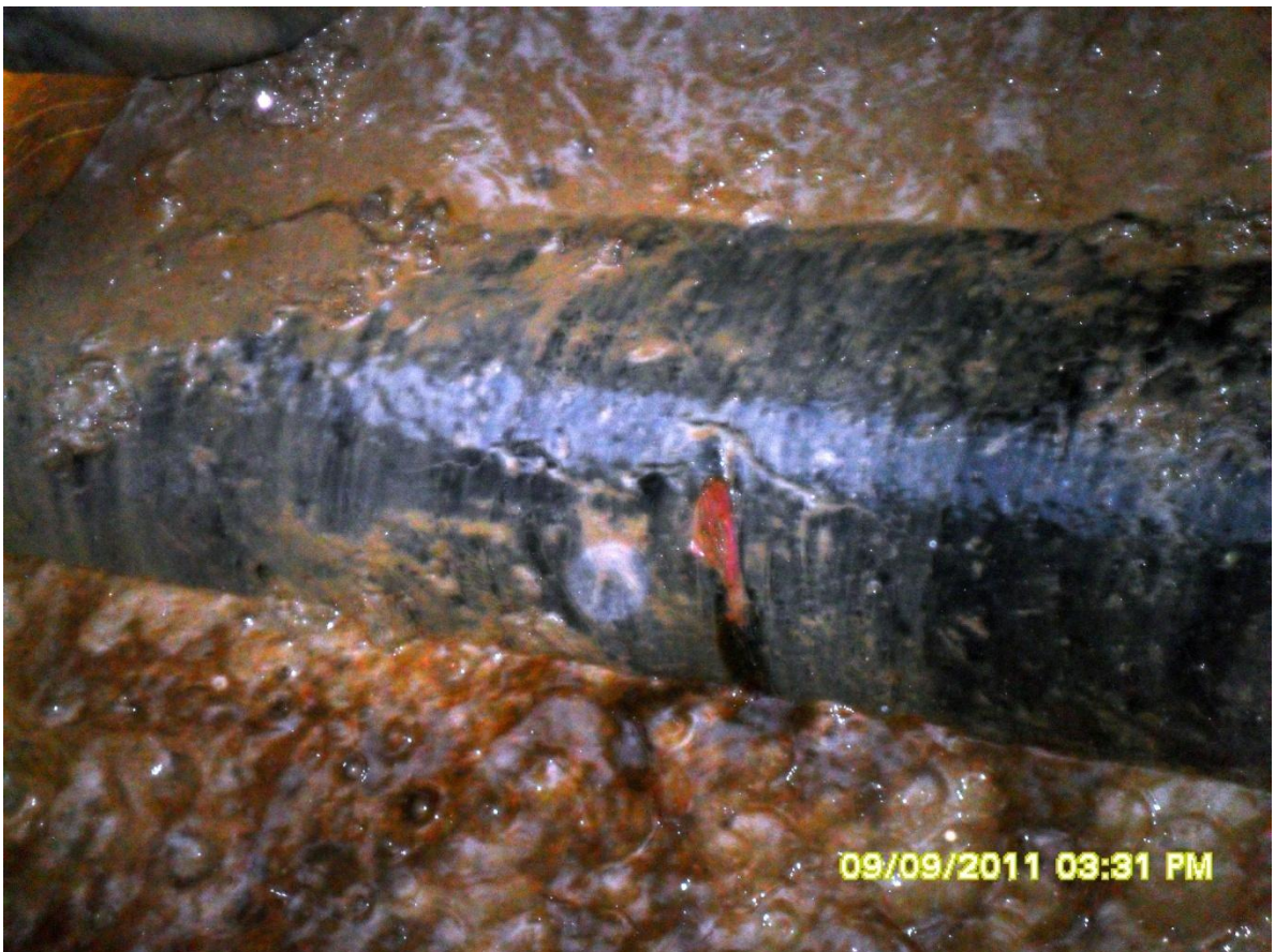
Close-up: Spill due to Hack saw cut on 14" Okordia – Rumuekpe Pipeline at Ikarama. Picture was taken during Joint Investigation of 9 th September, 2011
