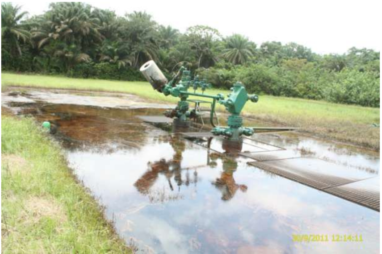
Overview: Part of the spill impact at Escravos Well3T at Ogidigben. Picture taken during Joint Investigation of 30 th September,2011
