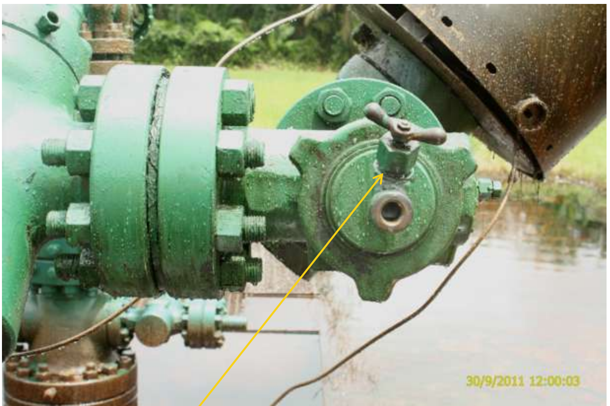
Close-up: Spill due to beanbox failure on Escravos Well3T at Ogidigben. Picture taken during Joint Investigation of 30 th September,2011
