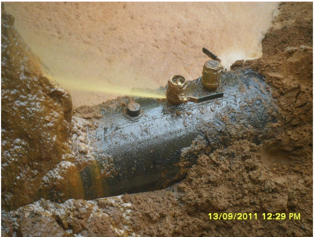
Close-up: Spill due to illegal fittings on 18" Assa-Rumuekpe Pipeline at Elele Alimini Picture taken during Joint Investigation of 13-14 th September, 2011
