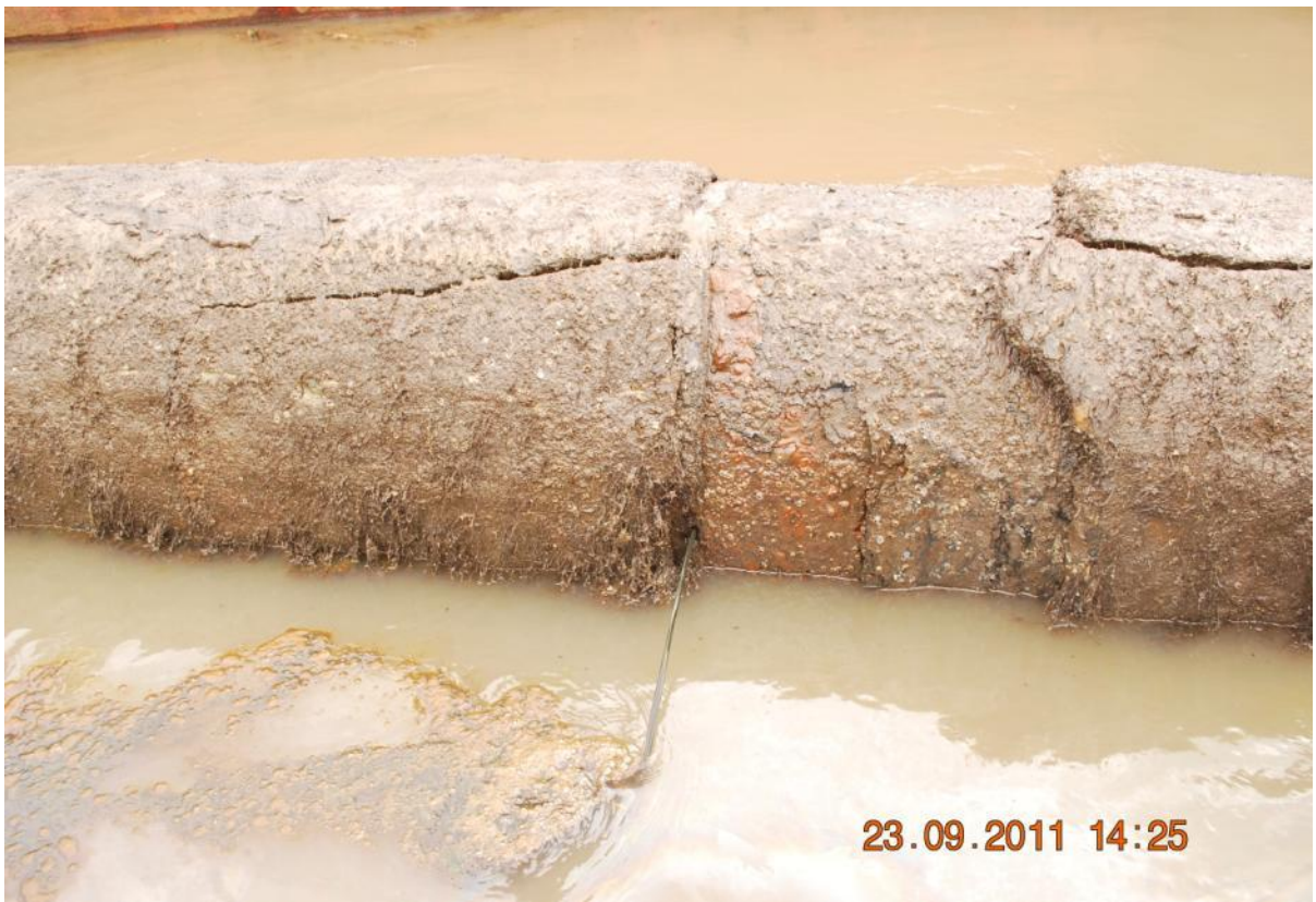
Close-up: Spill due to External Corrosion on 28 inch Trans Forcados Pipeline at Batan. Picture taken during Joint Investigation of 23 rd September, 2011.
