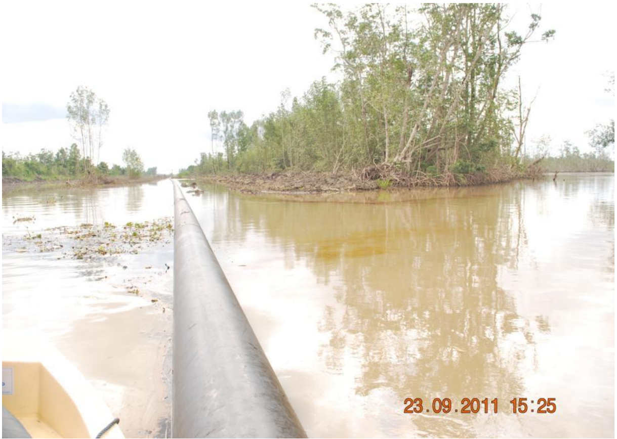
Overview: Part of spill impact on 28 inch Trans Forcados Pipeline at Batan . Picture taken during Joint Investigation of 23 rd September, 2011
