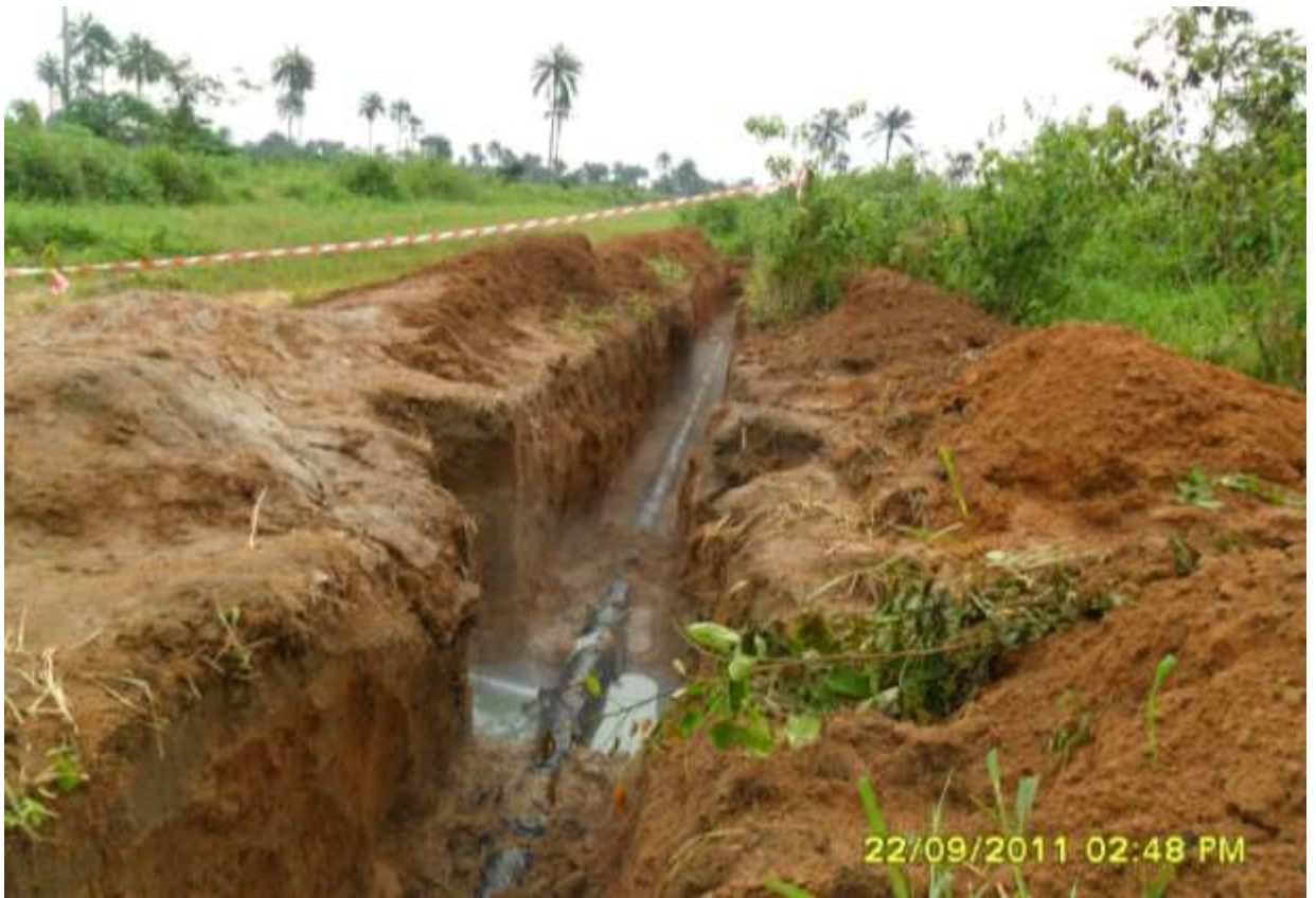
Overview: Part of the spill impact on 6'' Obigbo North-Ogale pipeline right of way at Ogale Picture taken during Joint Investigation of 22 nd September,2011
