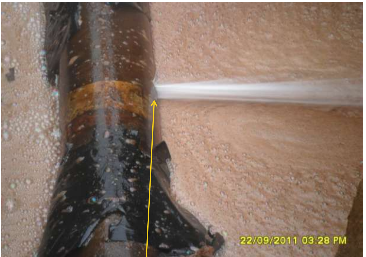
Close-up: Spill point due to hacksaw cut on 6'' Obigbo North-Ogale pipeline at Ogale. Picture taken during Joint Investigation of 22 nd September,2011
