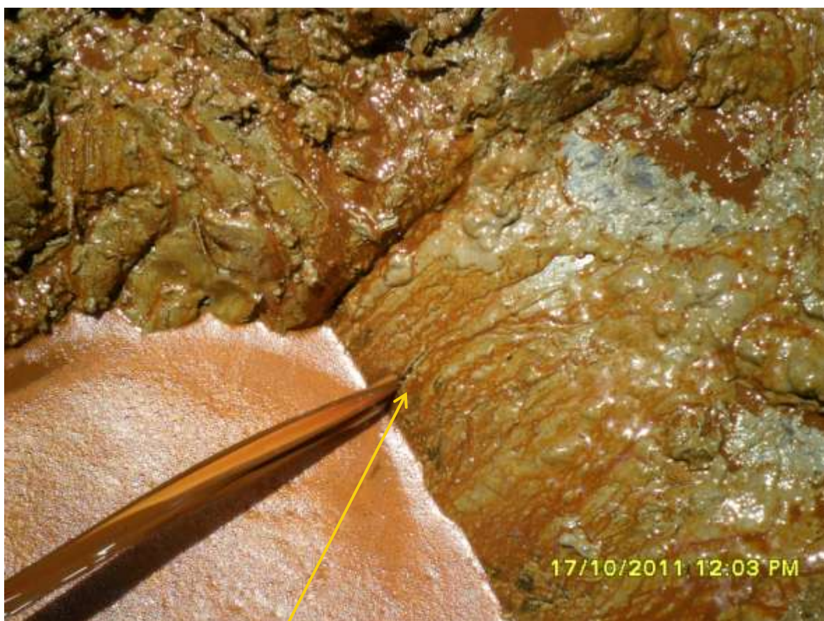
Close-up: Spill due to Hacksaw cut on 12" Adibawa-Okordia pipeline at Ikarama. Picture was taken during Joint Investigation of 17th October, 2011.
