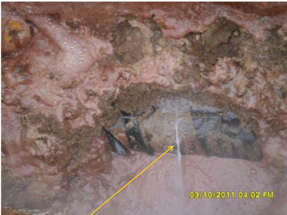
Close-up: Spill due hacksaw cut on 6" Obigbo North pipeline at Ogale. Picture taken during Joint Investigation of 3 rd October, 2011.
