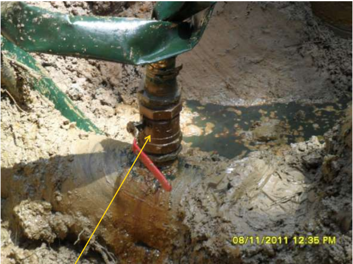
Close-up: One of three illegal fittings on 10" Diebu Creek pipeline at Oporoma. Picture was taken during Joint Investigation of 8 th November, 2011.
