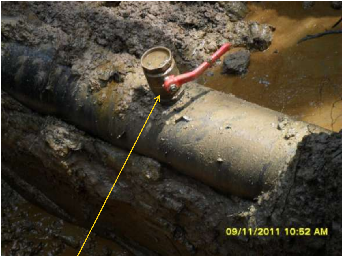
Close-up: One of three illegal fittings on 10" Diebu Creek pipeline at Oporoma. Picture was taken during Joint Investigation of 9 th November, 2011.
