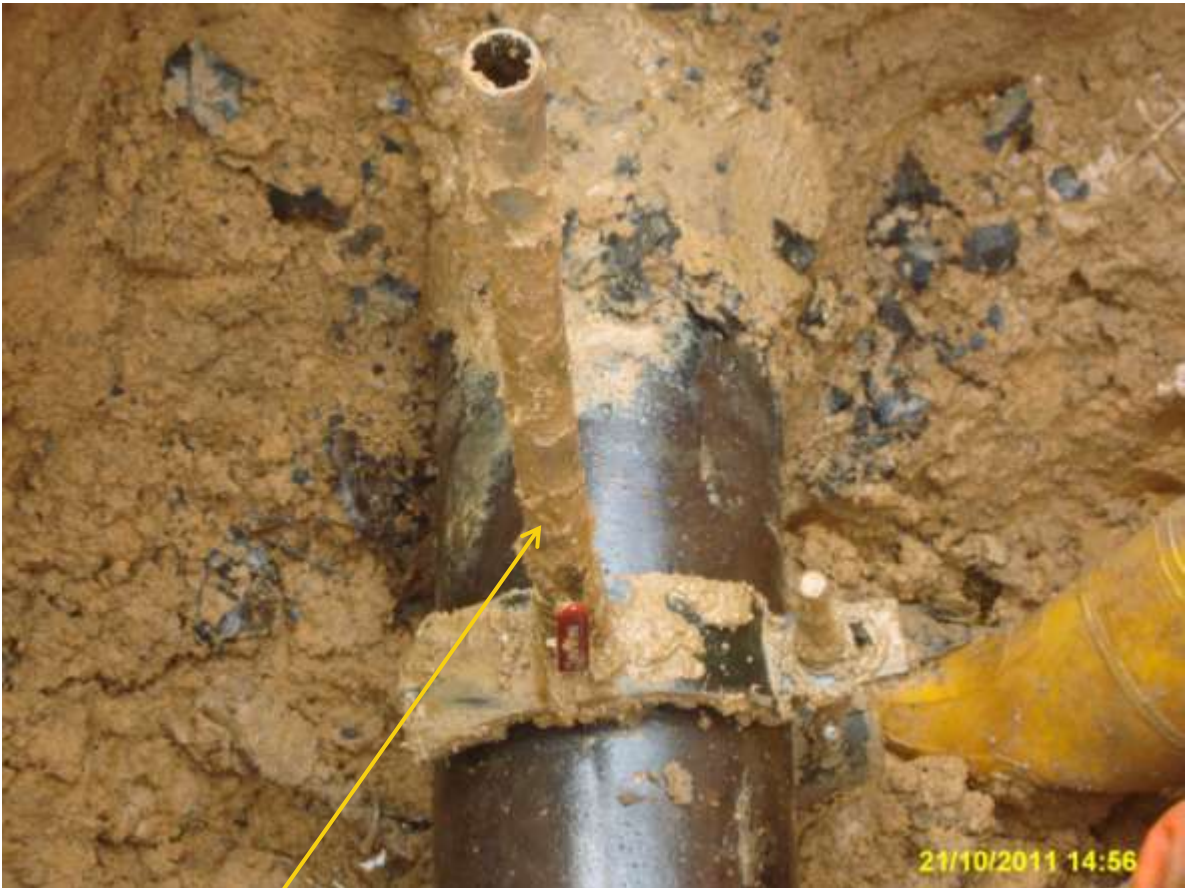
Close-up: Illegal fitting on 8" Umuechem-Nkpoku pipeline at Igwuruta. Picture was taken during Joint Investigation of 21 st October, 2011.
