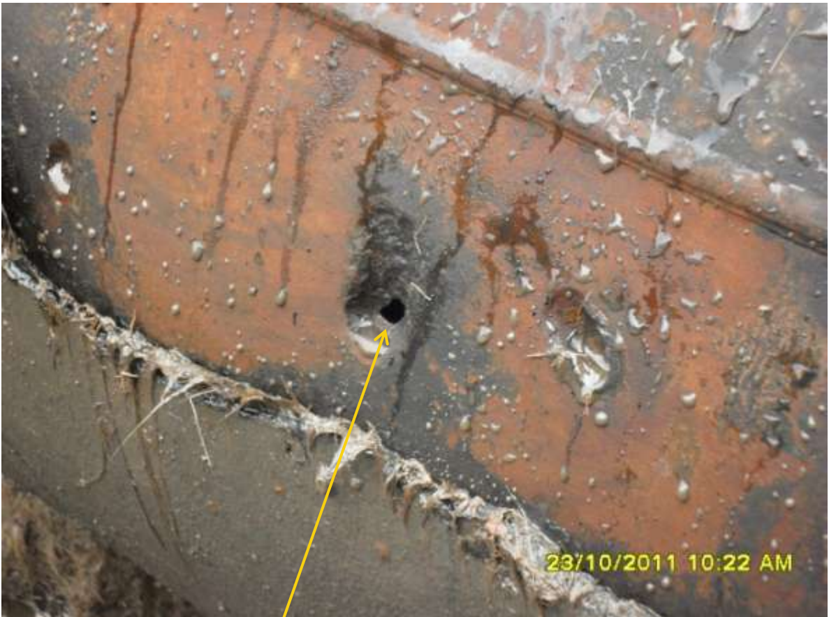
Close-up: Drilled hole on 20" Buguma-Alakiri pipeline at Bakana. Picture was taken during Joint Investigation of 23 rd October, 2011.
