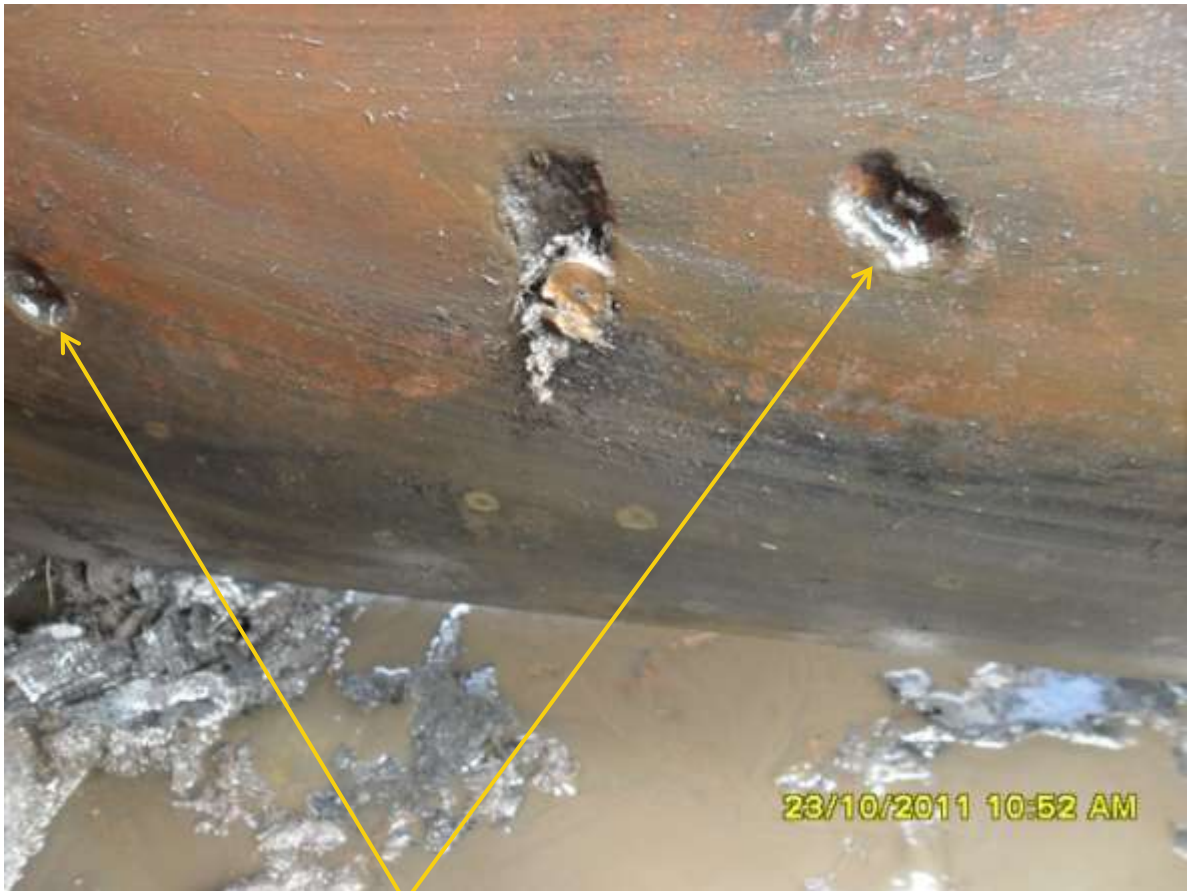
Close-up: Unsuccessful drill attempts can be seen after plugging the Drilled hole on 20" Buguma-Alakiri pipeline at Bakana.
