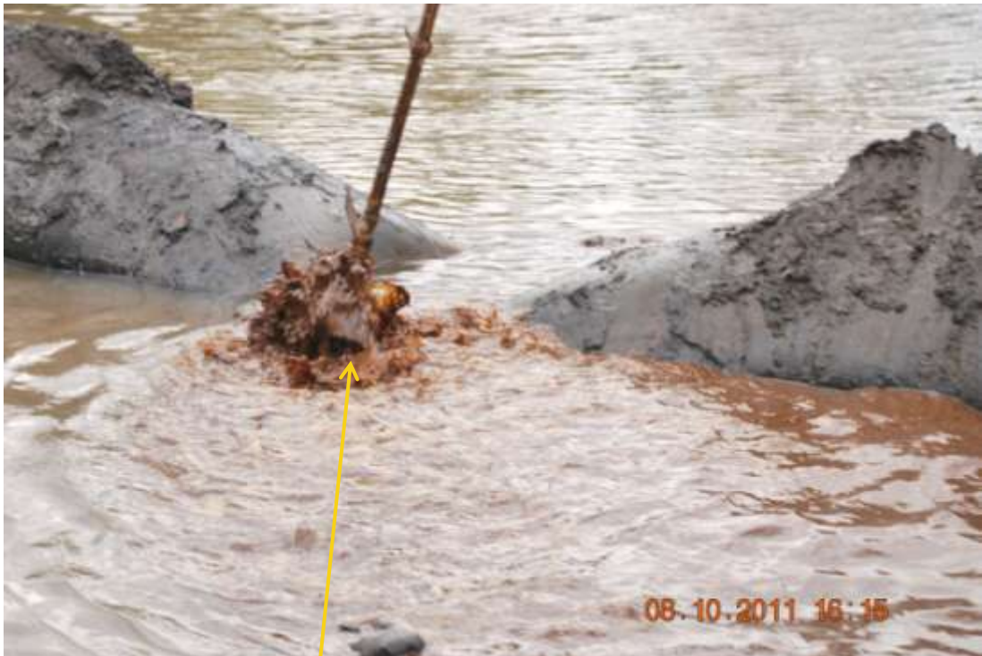
Close-up: Spill due to inward dent on 28" Trans Forcados pipeline at Batan. Picture taken during Joint Investigation of 8 th October, 2011.
