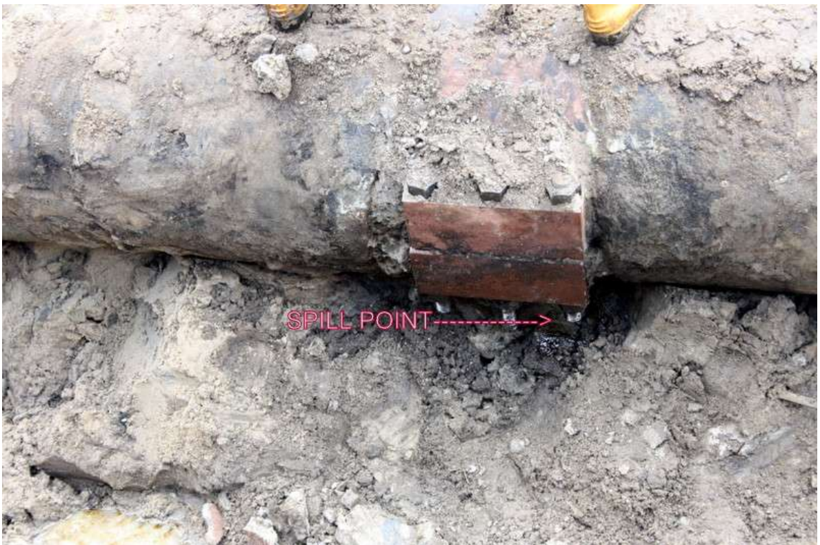
Close-up: Spill due to failed clamp on 20" Ughelli Pumping Station to Warri Refinery Petrochemical Company trunkline at Ugbomro. Picture taken during Joint Investigation of 13 th October, 2011.
