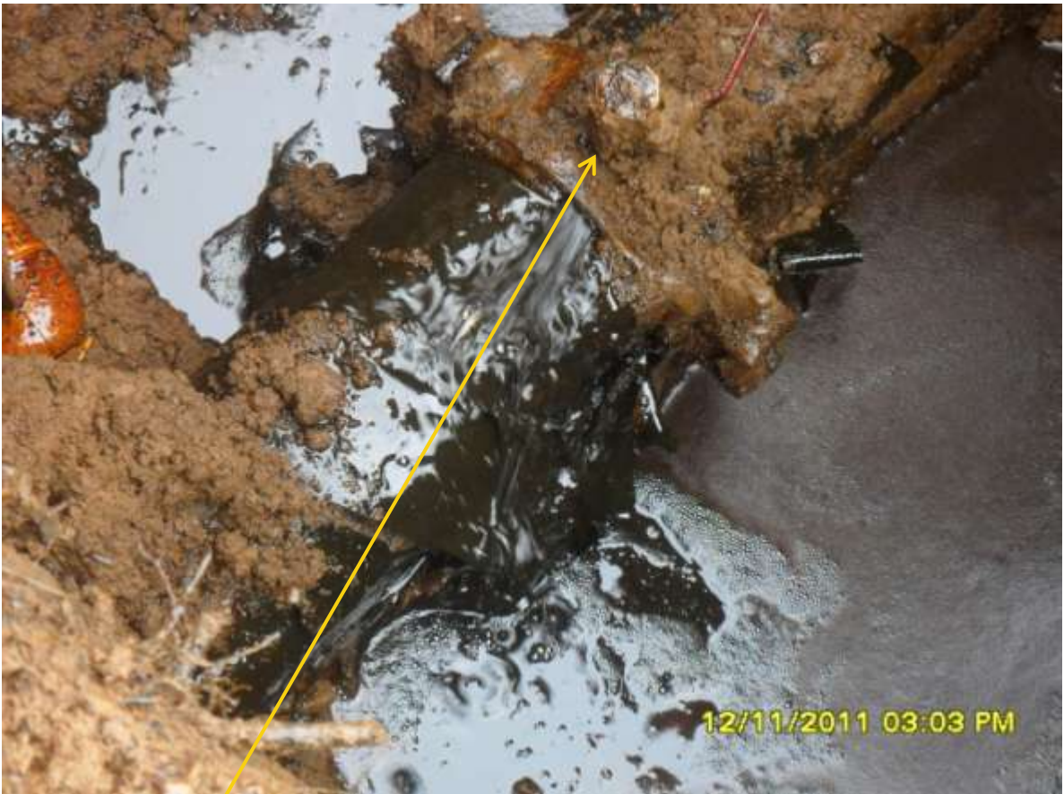
Close-up: Illegal fitting on 6" Obigbo North pipeline at Ogale. Picture was taken during Joint Investigation of 12 th November, 2011.
