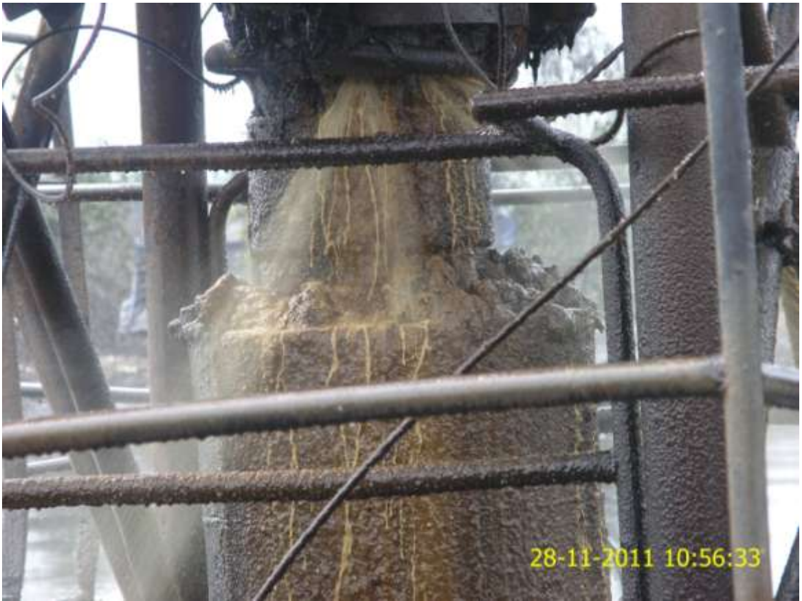
Close-up: Spill due to structural failure on Krakama Well 13 at Bille. Picture was taken during Joint Investigation of 28 th November, 2011.
